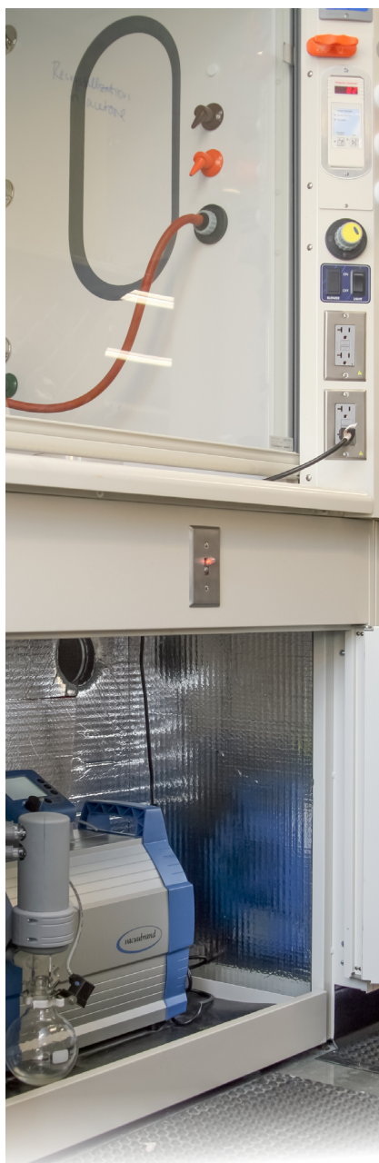
Local vacuum network pump under a fume hood.
